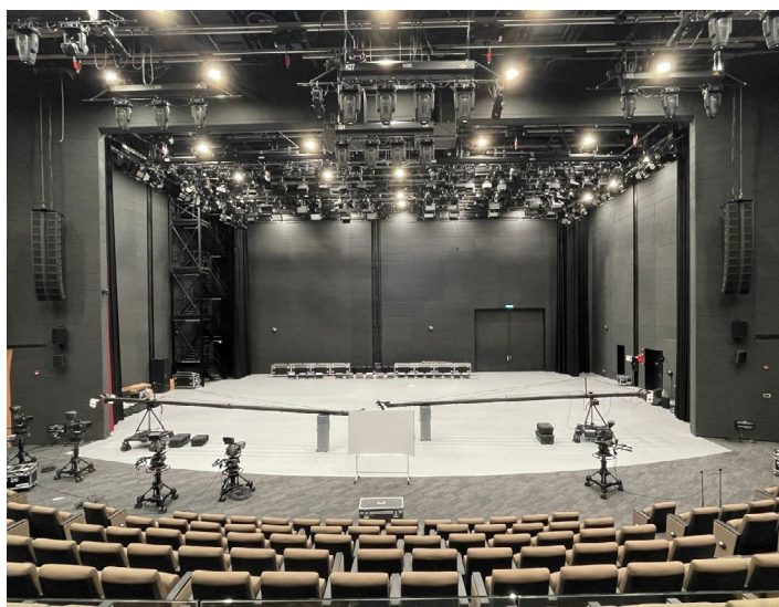
The LCR system consists of two L-Acoustics A15 boxes serving as centre-fill and a main L/R system of 12 Kara per side.
