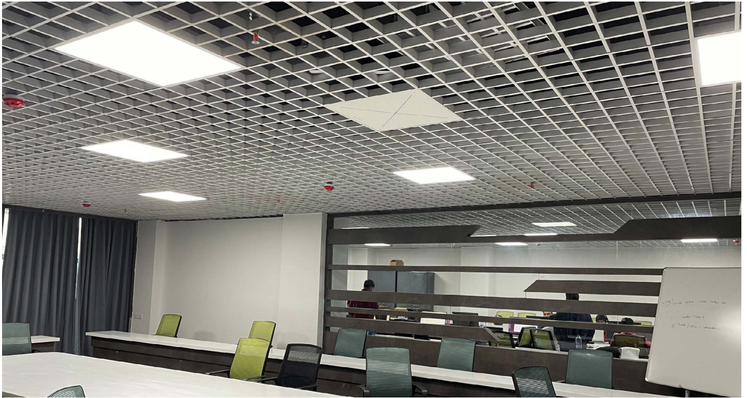
The Sennheiser TCC2 installation at an education facility in India.
