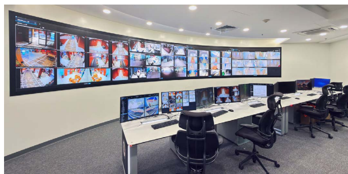
The curved COMET-C 1.2 videowall at the Security C&C.
