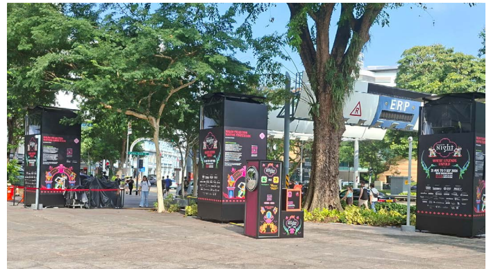
The projectors enclosed to protect them from the weather and the public.
