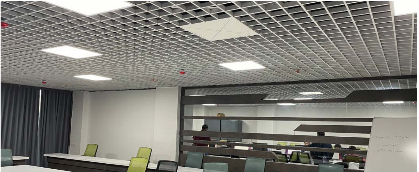
The Sennheiser TCC2 installation at an education facility.
